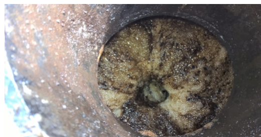
Fig. 4 Deteriorated TEG by foaming, inside the expansion vessel of the facility [14]
