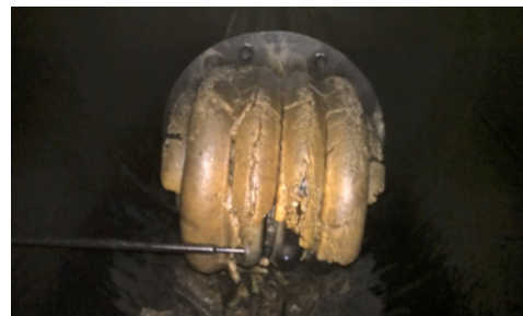
Fig. 5 Heat exchanger piping affected by salt crust [14]
